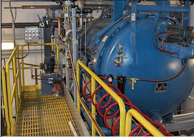
Figure 3-7. The groundwater collection and treatment system is an Interim Remedial Measure that is associated with the Willis Avenue sub-site. The system removes contaminants such as mercury and organic compounds from groundwater. (Source: Central New York Regional Planning & Development Board)
