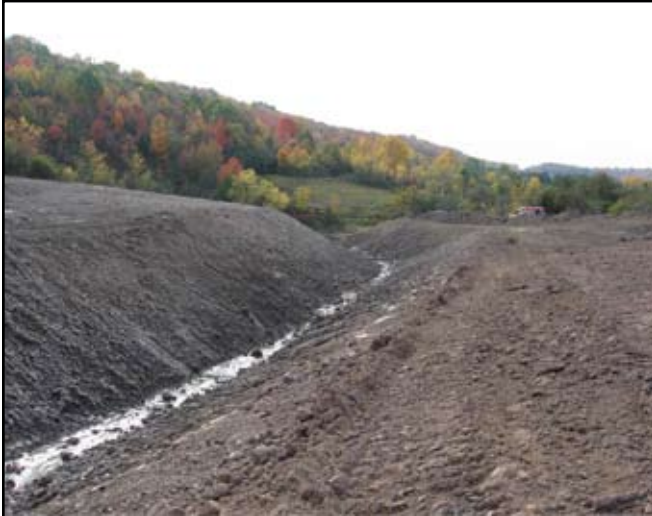
Figure 3-10. Pilot study activity at the mudboils. The photo shows Big Sink outlet, excavated to a depth of about 15 feet to maintain the water level in Big Sink at summer low levels. The work reduces seasonal fluctuations in the influx to Big Sink that are believed to contribute to mudboil activity. (Source: USGS)
