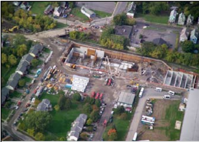
Figure 3-5. Aerial view of the Midland RTF while under construction during 2005. (Source: Onondaga County)
