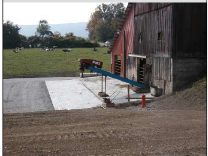
Figure 2-21. Post-BMP barnyard with concrete pad to reduce erosion and enhance animal waste management. (Source: OCSWCD)
