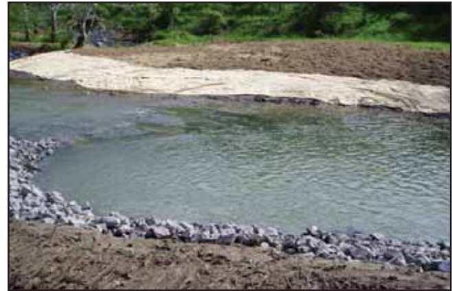
After: Boil up pool project to dissipate stream energy and prevent bank erosion.
