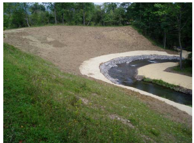
After Construction – New stream channel, streambank shaped and graded, and all areas seeded and Futura Matted or mulched.
