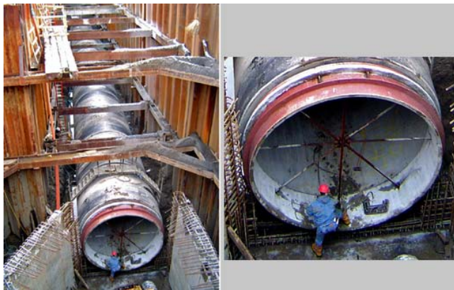
144-inch Conveyance Pipeline
